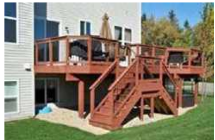
▲ A deck with two sets of stairs; only one is covered for egress.
