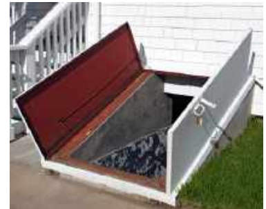
▲ Exterior egress in a basement is not covered.
